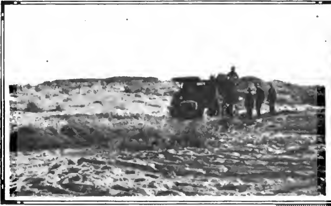
Building a road in the desert near Phoenix, Ariz., showing what the builders faced when they started work on the Arrow Weed Road
